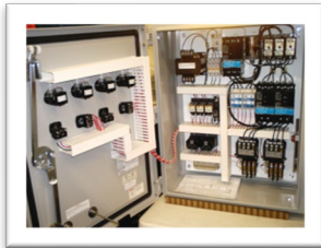
Clarifier Control Panel
