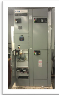
MCC and Power Panel
